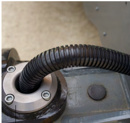
Excellent protection for exposed cables
