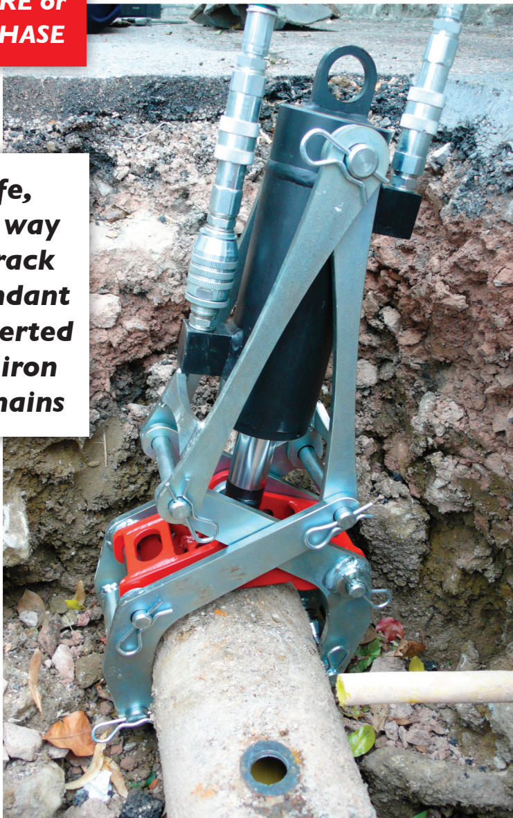
The Mini MACAW Pipe Cracker positioned on a 6" cast iron main prior to breaking out
